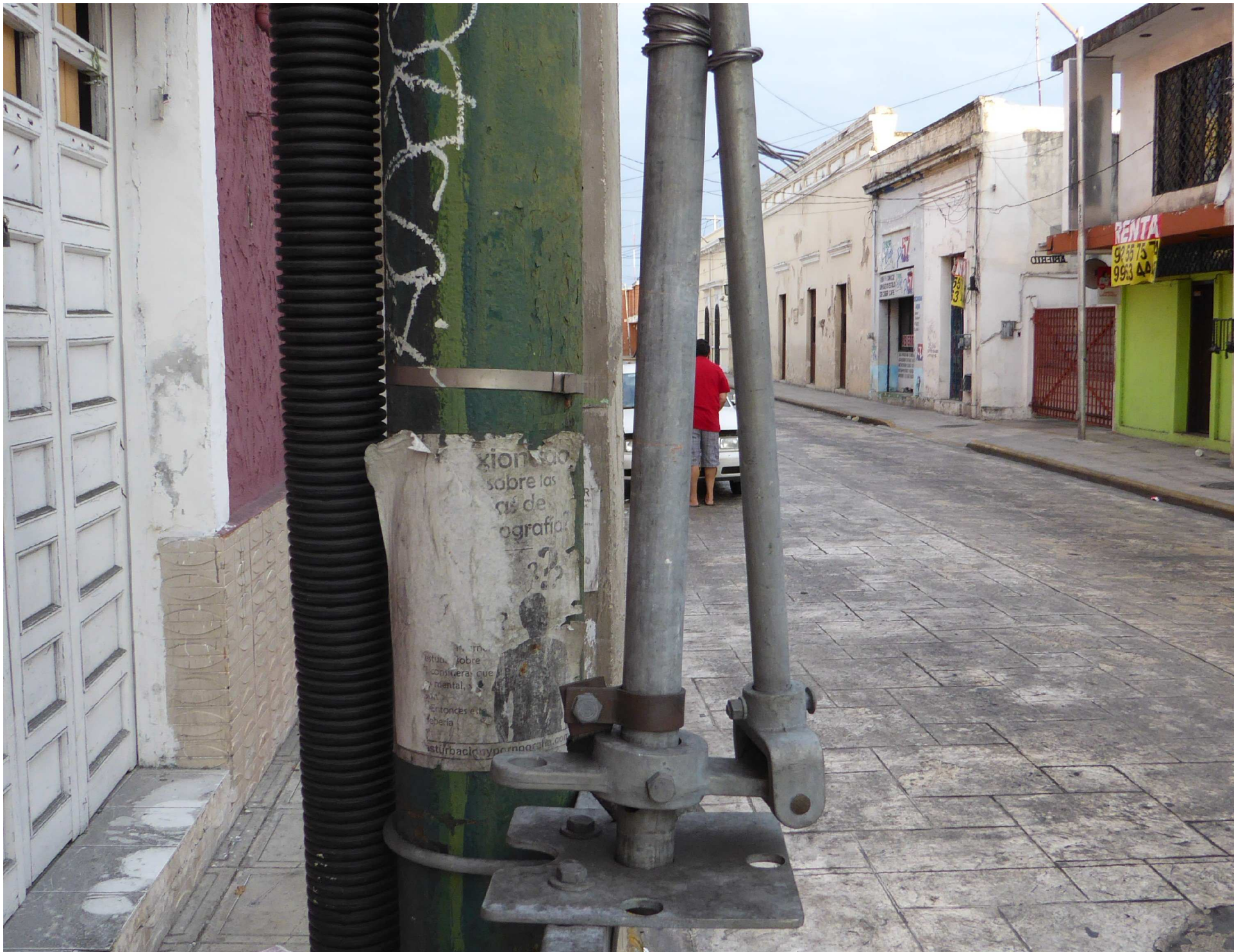
This unsecured lever is the disconnect switch for a 12,000 volt overhead line. Pulling it would, at least, take down an entire block, probably several blocks!
